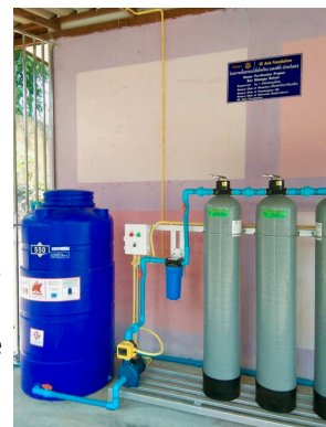
State of the art system newly installed
